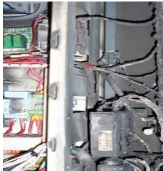
Electrical panel without a Firetrace System (after a fire occurred)
