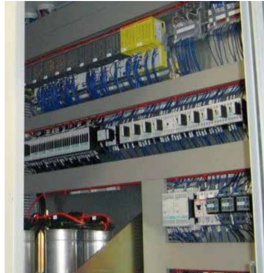
Panel fitted with a Firetrace System
